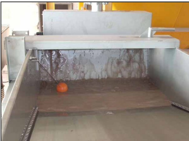
inlet sludge onto vacuum belt filter
